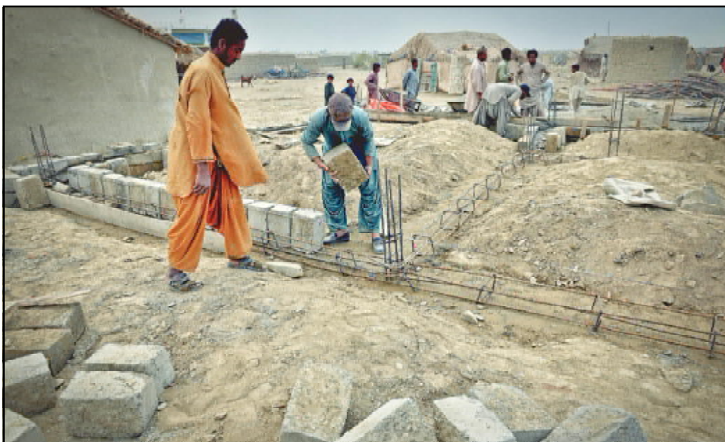
A labourer places a cement brick alongside an iron framework of a house that is being constructed in Malaar, Awaran. More than one year after the earthquake, reconstruction is still under way in the town.
